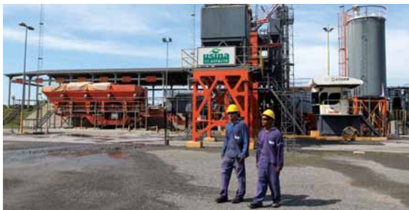
Asphalt Plant - Ecovias
